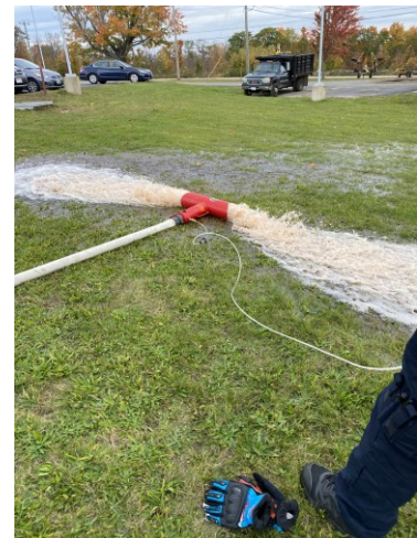
Fire Department flushing & testing apparatus
